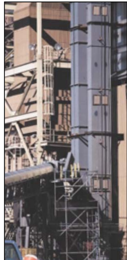
Figure 1: Bucket Elevator with Explosion Vents
