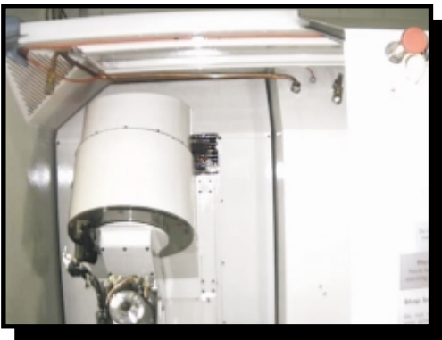
The machine's work area with Firetrace Detection Tubing, Discharge Nozzles and Manual Release.
