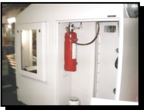
The 12 lb. Firetrace System installed in the back of the machine (with discharge piping visible).
