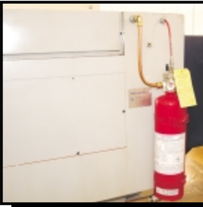
Firetrace Indirect Low Pressure System Installed Directly On The Machine
