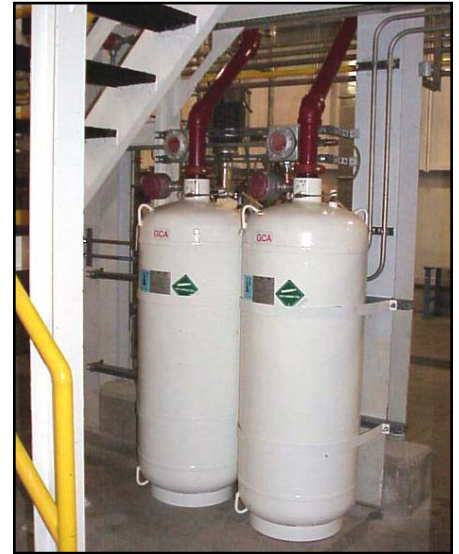
FM-200 System Protecting a Flammable Liquid Storage Facility
